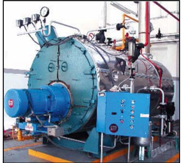
Model FD68CA250LM installed on a new packaged boiler system.
